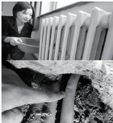
Heating Pipes/ Underfloor Heating Pipe Leaks
