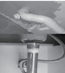
Water Supply Pipe Leakage/ Water Pipe Leakage
