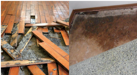
Leak Under The Floor
